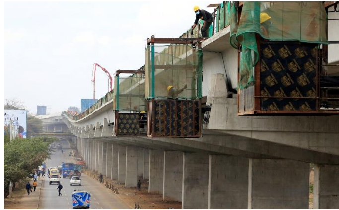
The Nairobi Expressway under construction in 2021. Photo: © picture alliance / REUTERS | Thomas Mukoya
